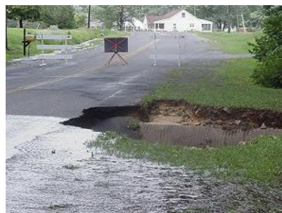
Photo Source: Caroline County Website: https://www.carolinemd.org/227/Road-or-Bridge-Closures
